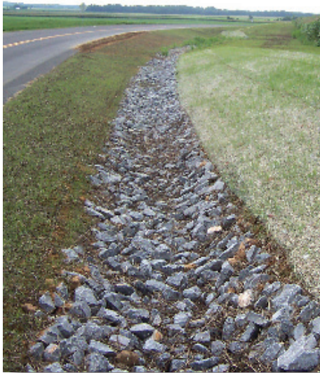
The rock is a little thin along this ditch, but could be acceptable because of the lack of visible channel erosion. Ditches should be monitored so that rock or other protective controls can be added if erosion becomes a problem.
