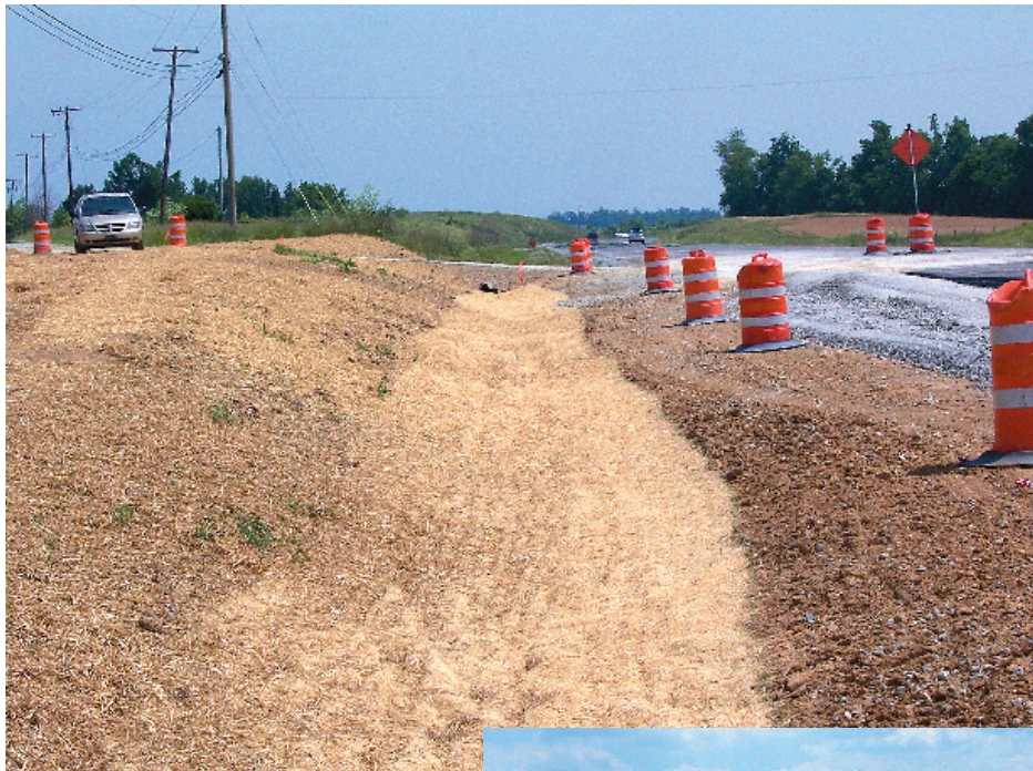
Here is an excellent construction of triple-seeded ditch with excelsior blanket. Ditches should be stabilized, seeded, and mulched immediately after construction.
