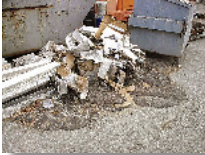
Here is an example of poor waste management. Construction contractors should provide appropriate waste disposal containers, and employees should be instructed to use them.
