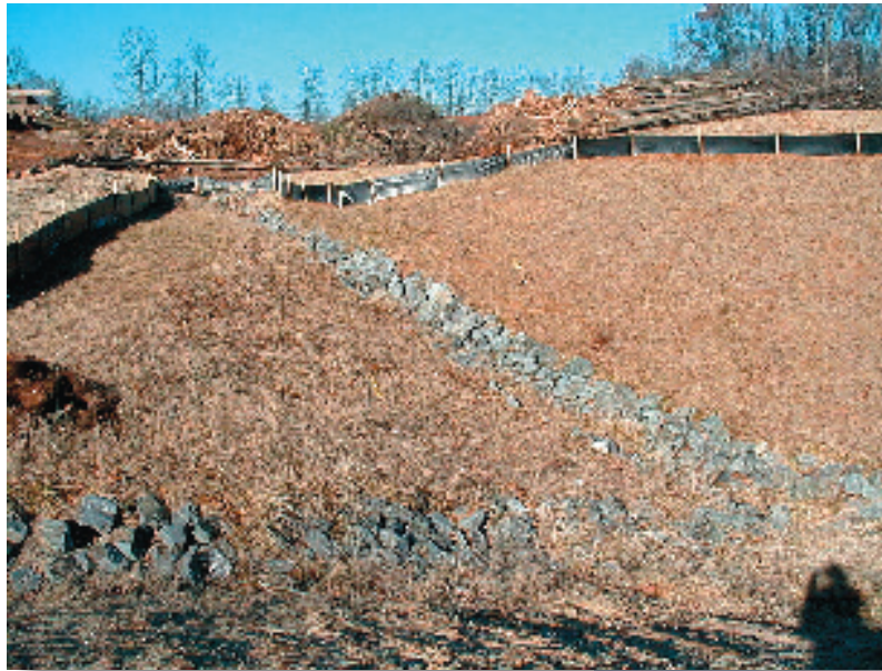
Install silt fencing, sediment traps, and stabilize ditches before clearing and grading. Make sure stakes are on the downhill side of the silt fence!
