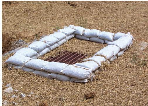
Inlet protection berm constructed of half-filled stone bags. Use #57 rock, overlap bags to eliminate large openings and rapid flow-through. Construction-grade bags of netting material—similar to onion bags—can also be used.
