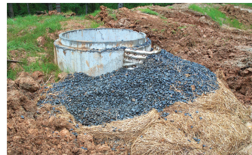
Side slot in drop inlet protected by half-round section of corrugated metal pipe with one-inch holes, held in place by stone berm. This modification can also be used on sediment basin outlet risers.
