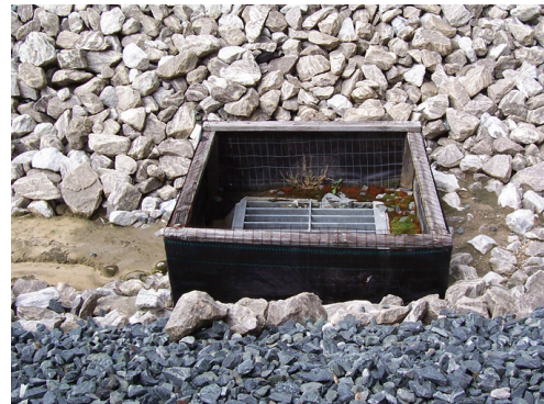
Silt fencing can be used as an inlet protection device if flow volumes and velocities are low. When using a silt fence frame to construction in inlet protection dike, add wire reinforcement and cross-bracing to prevent collapse in areas of heavy flows.
