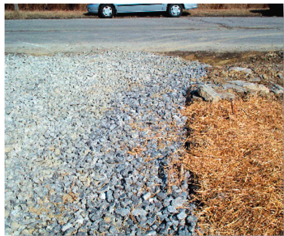
The construction exit will be one of the first things an inspector sees at the construction site and is often a good indication of how other controls are installed and maintained.
