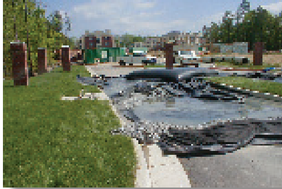
This shows a dewatering sediment filter bag (center) in use at residential construction site. Muddy water pumped into the bag is physically filtered, with clear water passing through the bag fabric. Pumping muddy, unfiltered water directly into curb drains (center left) or surface streams constitutes a direct KPDES permit violation.
