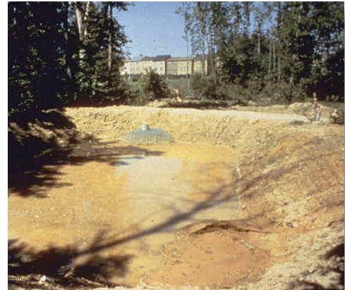
This is a well-constructed sediment basin. Note the rock flow restrictor around outlet riser, which filters and detains inflows. Basin sidewalls should be seeded immediately after construction.
