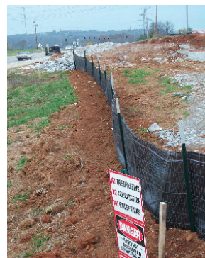
Super (wire reinforced) silt fence in the foreground, supplemented by rock sediment barrier (background). Use rock or other sediment barriers when appropriate.
