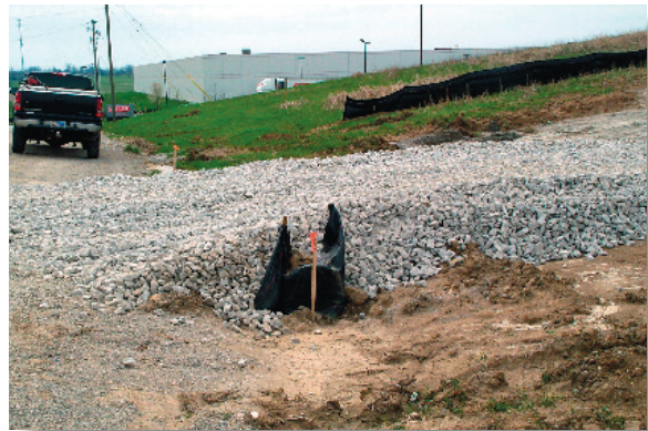
A well-maintained construction exit keeps mud off the pavement and helps to reduce potential legal liability.
