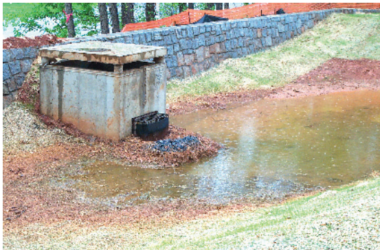
This outlet riser intake hole has been modified with a “half round” section of pipe with 1-inch holes on 6-inch centers and rock berm. This temporary dike provides additional detention during the construction phase, which improves soil removal.
