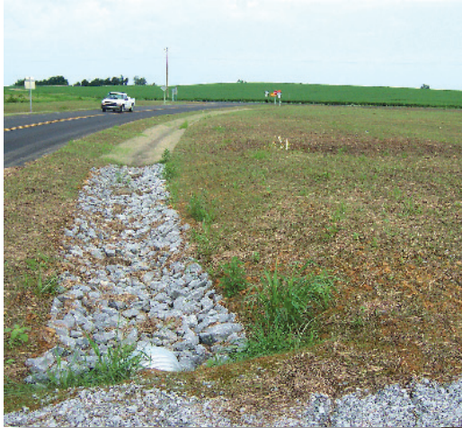
Here is a good example of rock-lined ditch. The seeding is a bit too thick on the side slopes.
