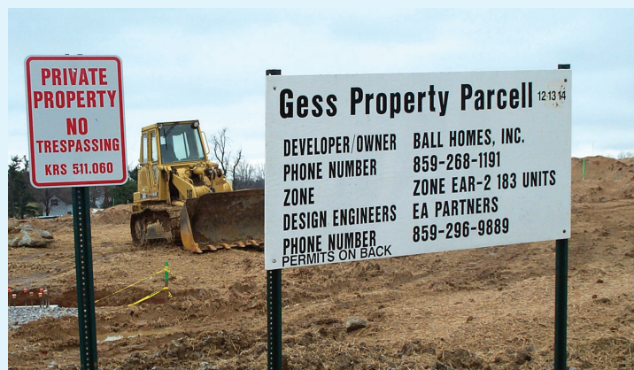
Listing the construction site operator and posting applicable permits makes it easy for inspectors to quickly check whether or not a site is in compliance with various state and federal regulations.
