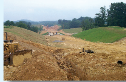
Linear construction sites require special attention to drainage within—and into—the construction zone.
