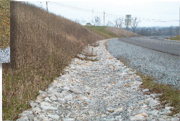
This shows a very good stabilization of slope and ditch on highway project. Note the mix of large and small rock, which helps fills voids and deters undermining.
