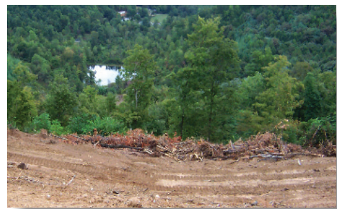
Brush cleared from the site used as a temporary downslope sediment barrier. Make sure barrier intercepts and ponds up muddy runoff. Remove when grass is established.
