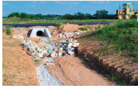
Poor placement of outlet dissipator rock; poor ditch lining (no grass, mulch, or blanket); poor slope protection.
